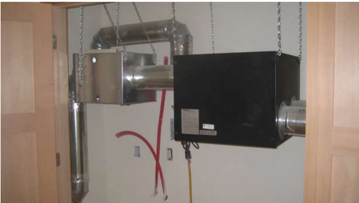
Image 4: Ventilation system fits in the closet (Photo credit: Joe Gransee-Bowman).
